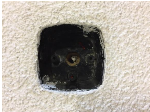
Photo 7 – Built-in socket and transition to wall – after test
